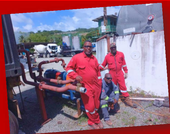
In January 2025 the team travelled to the sister Isle of Tobago to execute the project: Modification of Warner Construction Hot Mix plant to accommodate the use of TLA/AC for the Tobago Airport project.
